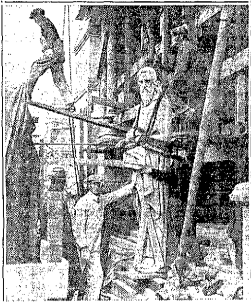
STATUE OF ST. ANDREW , weighing four tons, is pictured just before workmen hoisted it to its niche atop the western facade of the Cathedral of St. John the Divine in New York. It is the third statue to be placed on the facade, which has niches for seven more.
